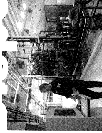
Plasma Arc Destruction Unit
